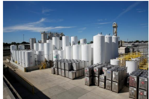
Solvent storage tanks at Gage Products’ 12-acre campus in Ferndale, Michigan.
